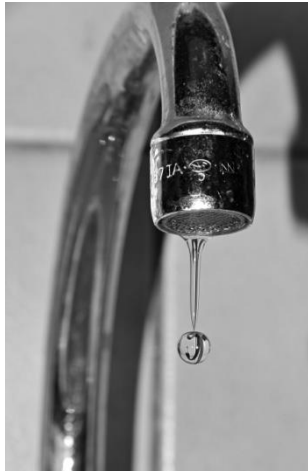
Figure 46 Tap with faucet aerator
