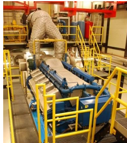
Figure 82 Diesel generator, source:
