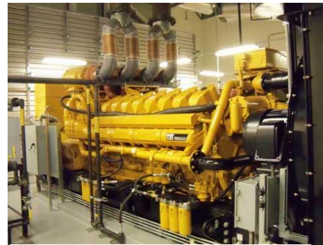
Figure 84 Dual fuel CHP as EPS
