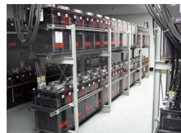
Figure 86 Data center UPS battery
