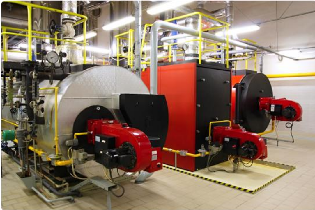
Figure 9 Hospital Boiler room for Steam production
