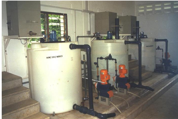
Figure 81 Water chlorination plant
