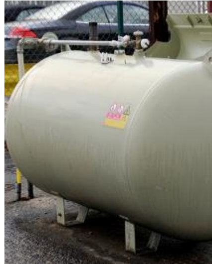
Figure 13a Liquid gas storage tank
