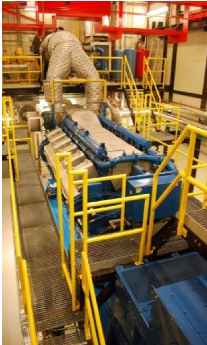
Figure 18 Dual Fuel CHP unit 4,1 MWe
