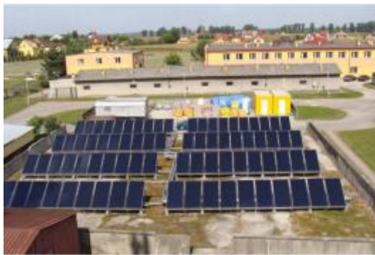
Solar collectors field
