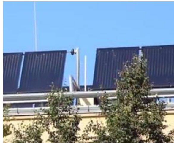
Solar collectors on the roof of hospital building
