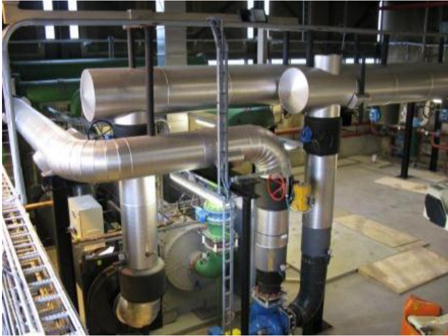
Figure 16 Chilled water plant
